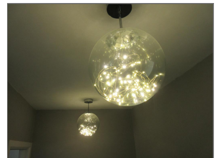
Landing Light Fittings
